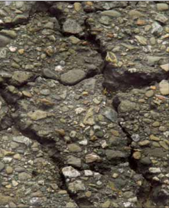
Left, the freeway pavement currently suffers from wear and tear, causing cracks, dips and potholes in some sections of I-680. Caltrans plans to repair damaged areas with rubberized asphalt in 2009, but not to pave the entire freeway as Alamo and Danville residents have requested.
