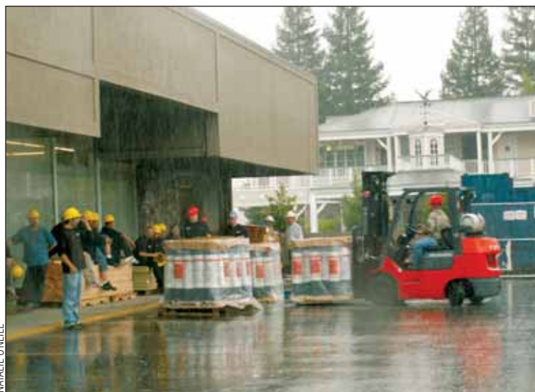
Shames Construction employees work alongside electricians from Foley Electric, despite unusually wet circumstances, to help prevent further delay of the Home Depot-Yardbirds opening.
