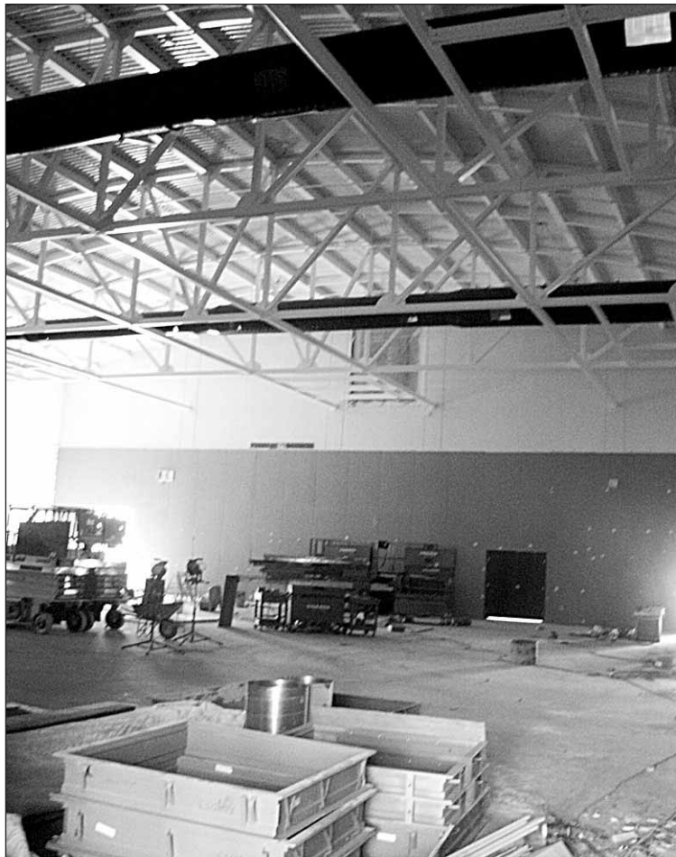
The Diablo Vista Middle School gymnasium will be finished and ready next school year, and it will be open to Danville residents, as part of a joint use agreement between the school district and Danville.
