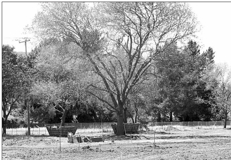
The project on Hansen Lane near Osage Park in Danville is transplanting eight trees as the land is divided into lots for the new homes.
