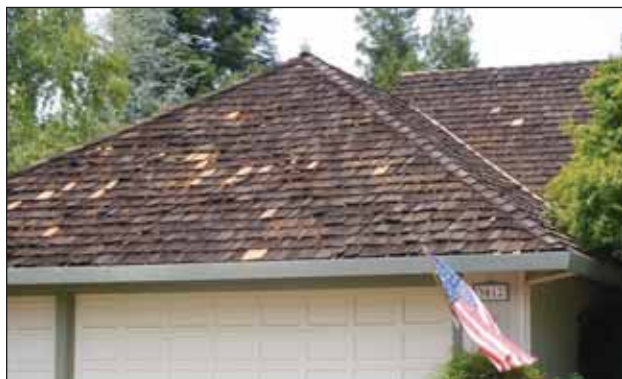
Wood shake shingles on a Bryan Terrace home begin to darken and decay; this roof has been patched in places. Shake roofs generally last 15-25 years.
