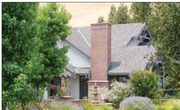
Tri-laminate asphalt shingles like these are not permitted by the homeowners association for aesthetic reasons though residents say they last longer and are safer than shake.
