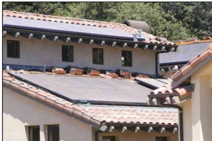
Two 4-by-10-foot solar panels on the roof instantly convert sunlight into electric power; if the homeowner is on vacation, the PG&E meter actually spins backwards.
